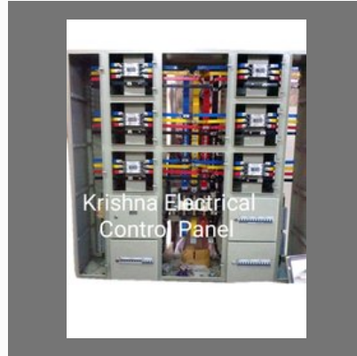
Distribution Control Panel
