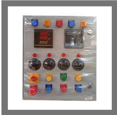
Paper Plate Machine Control Panel
