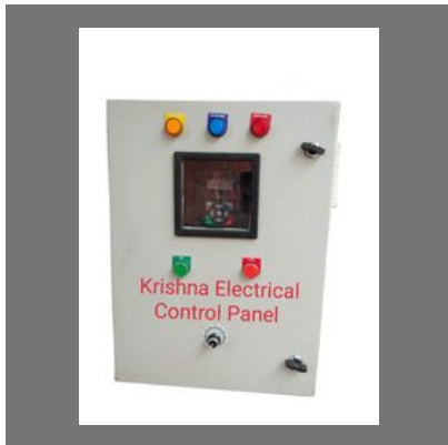
Variable Speed Drive
